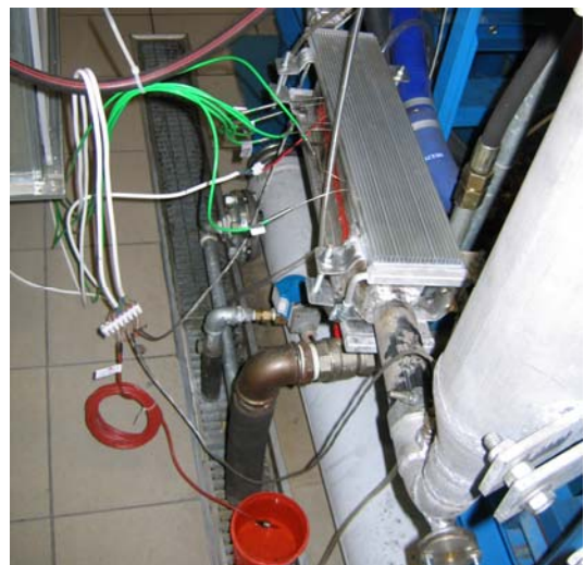
Fig. 2 Picture of the thermoelectric generator mounted on exhaust system of self-ignition engine.
